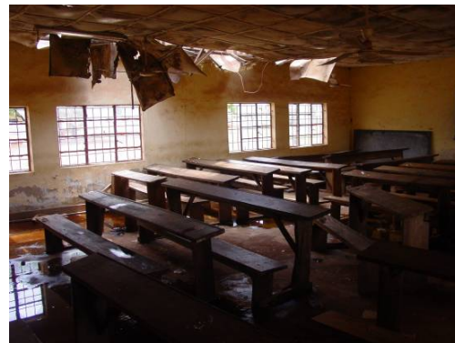
The most disturbing example of building dilapidation: a completely collapsed roof in the education faculty. Loose pieces of corrugated sheeting blow dangerously in the wind, on the exterior.
