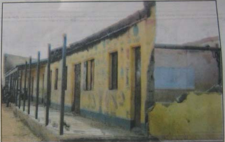
•The burnt Ungwan Muazu Primary School building
